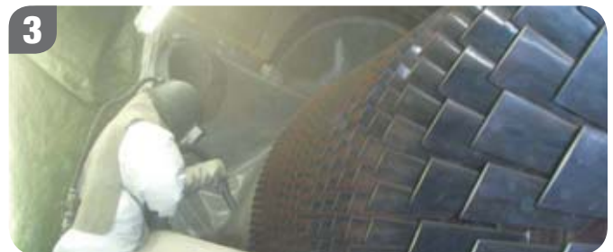
Grit blasting removes old coatings, rust and other fouling elements from the surface.
