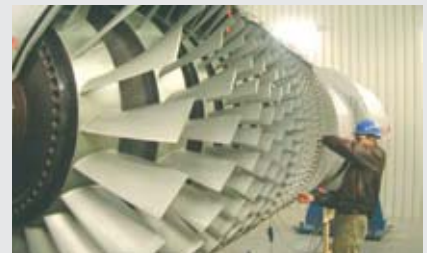
On-site coating can eliminate the need to remove vanes or disks—there's no need to de-stack and later re-stack compressor blade disks. Instead, critical components stay on-site and are ready for use without shipping delays.
